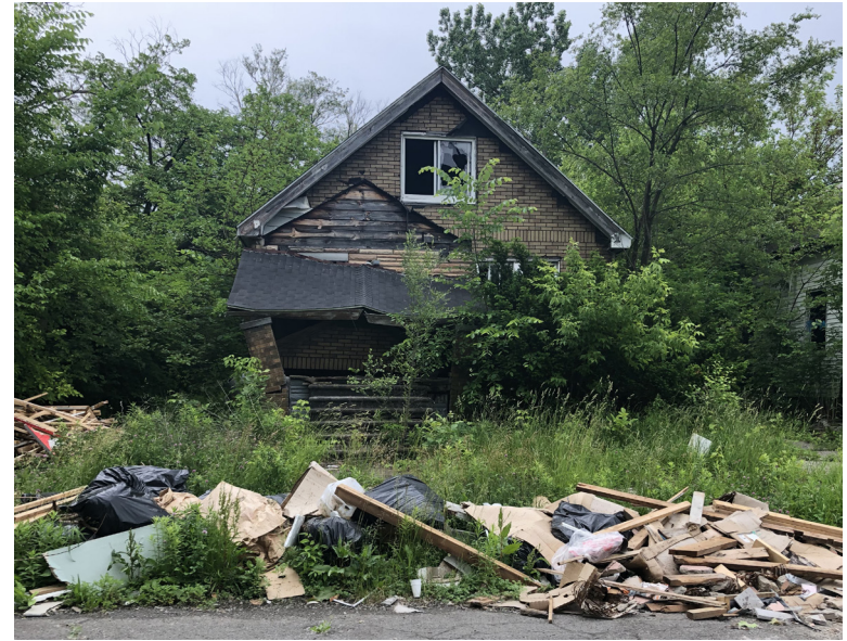
Figure 5-2: Example of dumping in Eden Gardens.
