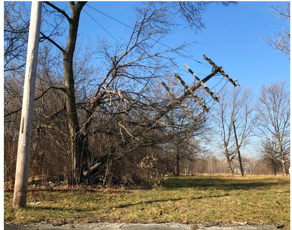
Figure 2-2: Downed power lines caused by unstable trees in Detroit.
