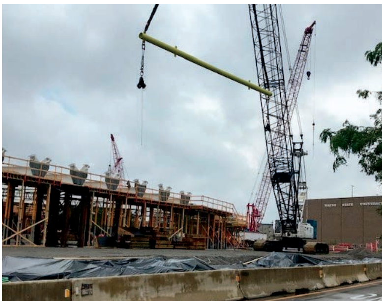
Assembly of the central arch is taking place amid a thicket of cranes in a parking lot near the WSU Law School. It will be rolled across I-94 sometime in 2021.
